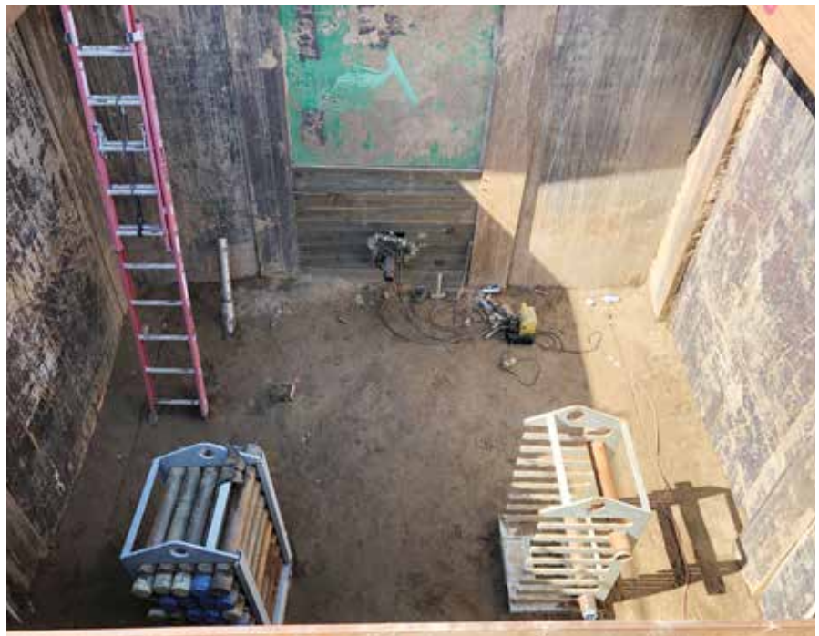
Figure 5. Pilot tubes entering reception shaft and being removed as 20-inch casing is advanced. Pilot tubes entered reception shaft precisely on line and grade.
