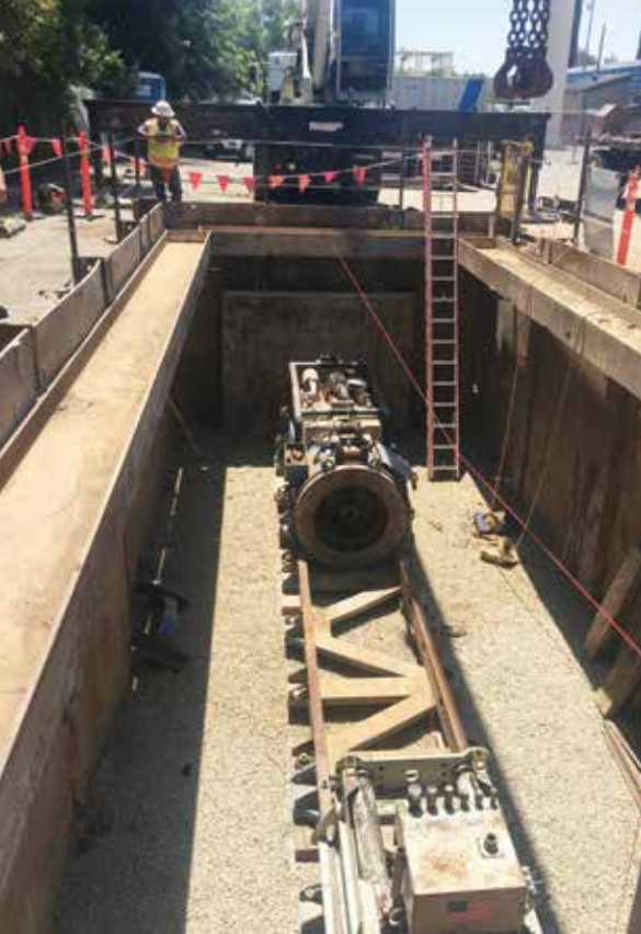
Figure 3. Auger boring rig set in the launch shaft with pilot tube guided boring equipment in foreground. Installation of 250 feet of guided pilot tubes took two hours.
