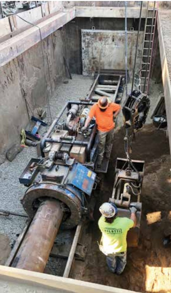
Figure 6. Auger boring installation of 20-inch casing beneath two sets of UPRR tracks.
