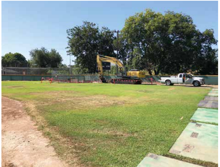
Figure 4. Reception shaft located in community baseball park's centerfield. Careful coordination with local baseball league was required and construction schedule was restricted to minimize construction impacts on community.
