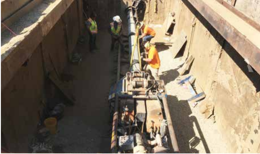
Figure 7. Installation of 12-inch cement-mortar lined and coated steel carrier pipe inside the 20-inch casing installed with guided boring took three days.
